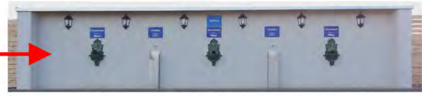
5 x Cassette toilet - disposal
